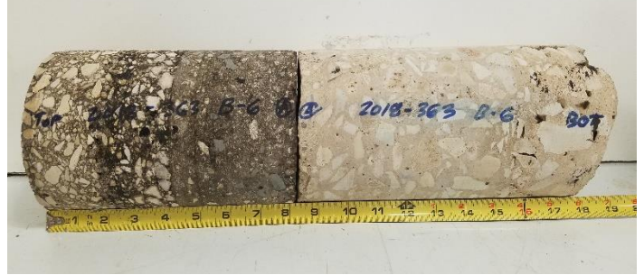
Asphalt and Concrete Core from Boring B-6 North of Broadway St and Appler St Intersection At Southbound Left Lane
