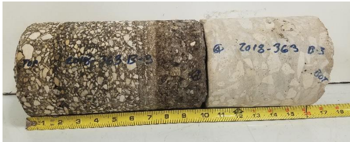
Asphalt and Concrete Core from Boring B-3 North of Broadway St and Funston Pl. Intersection At Southbound Left Turn Lane to Funston Pl.
